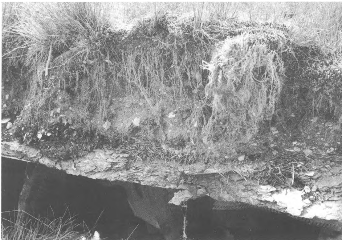
Figure 4. The collapsing roof of a traditional “sod” roof log cabin on the Pavilion reserve. This structure is reported to be over 80 years old and has only recently begun to decay because it was abandoned and unheated in the winter. Roof construction techniques are probably very similar to those used to roof pithouses. Note the use of pine needles and pine bark slabs at the base of the earth covering in the detail photo. Wood shakes have probably replaced poles as construction material used between the roof cross beams and the pine bark.
